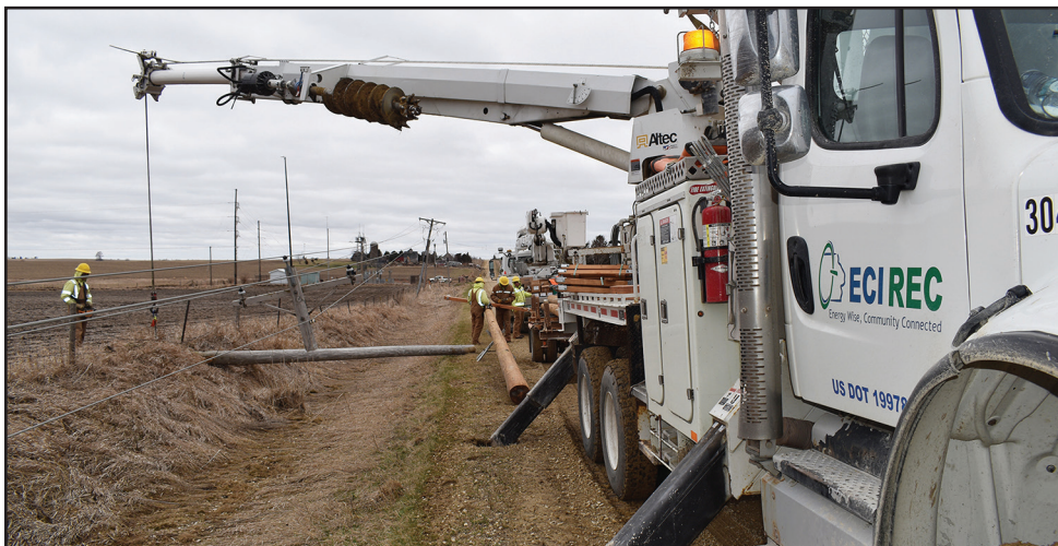
Personnel from East-Central Iowa REC prepare to replace a pole just east of the Clarence substation following the March 31 severe storm.
