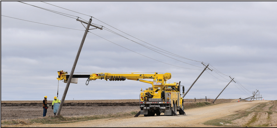
A Butler County REC crew prepares to repair a section of line in Cedar County northeast of the Clarence substation.
